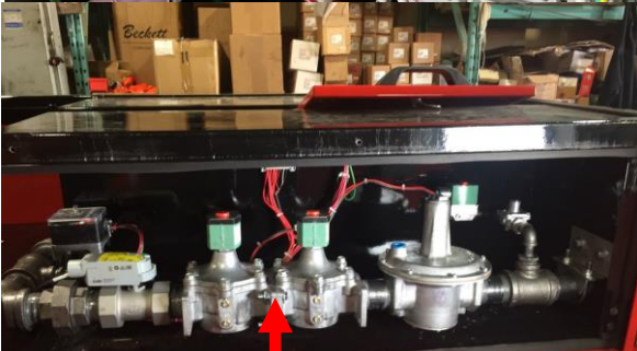
Main burner Gas Valves
